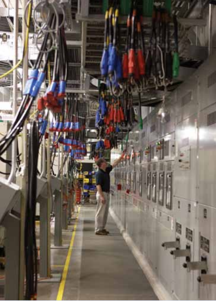
Eaton's Witness Test Centers allow you to see your large multi-module system tested before it's deployed.
