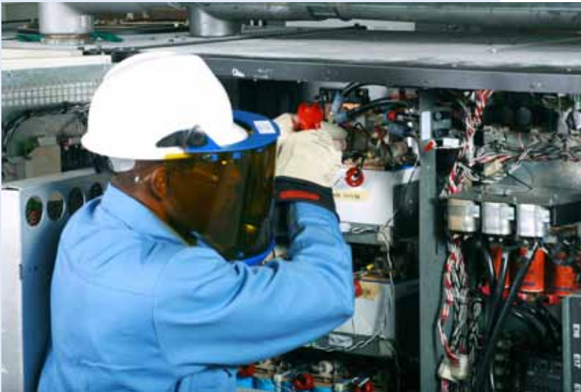
Eaton provides a 24x7 call center and has 240 service technicians across North America (See page 41)
